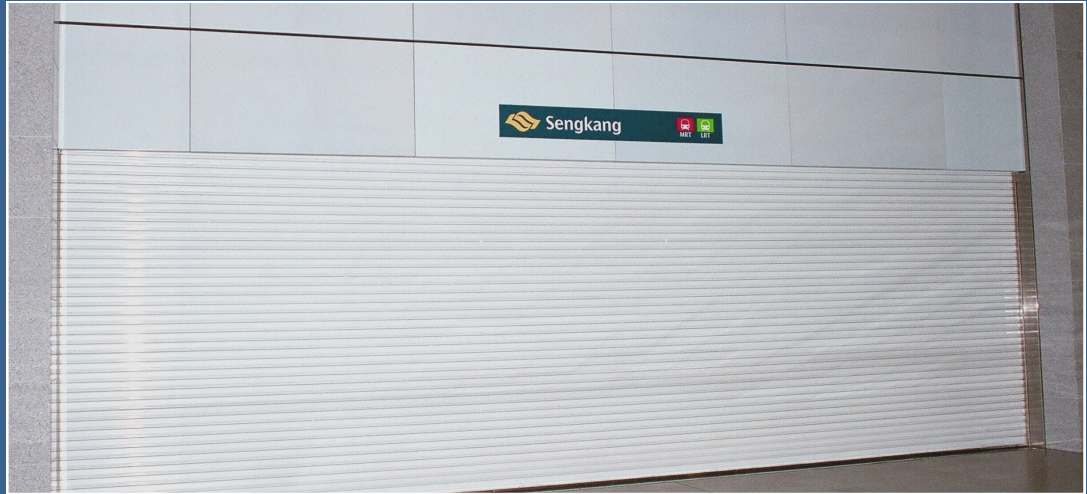
10m wide fire shutter at Seng Kang MRT Station, Singapore
